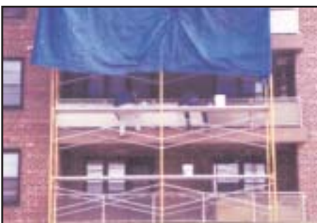
Glass panels enclosing apartment balconies being primed with Bulls Eye 1-2-3 to insure adhesion and extended life of the topcoat in all kinds of weather.
