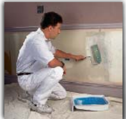
Joe Donaway of Joe Donaway Wall-covering Installation, using DIF GEL to remove clay adhesive.
